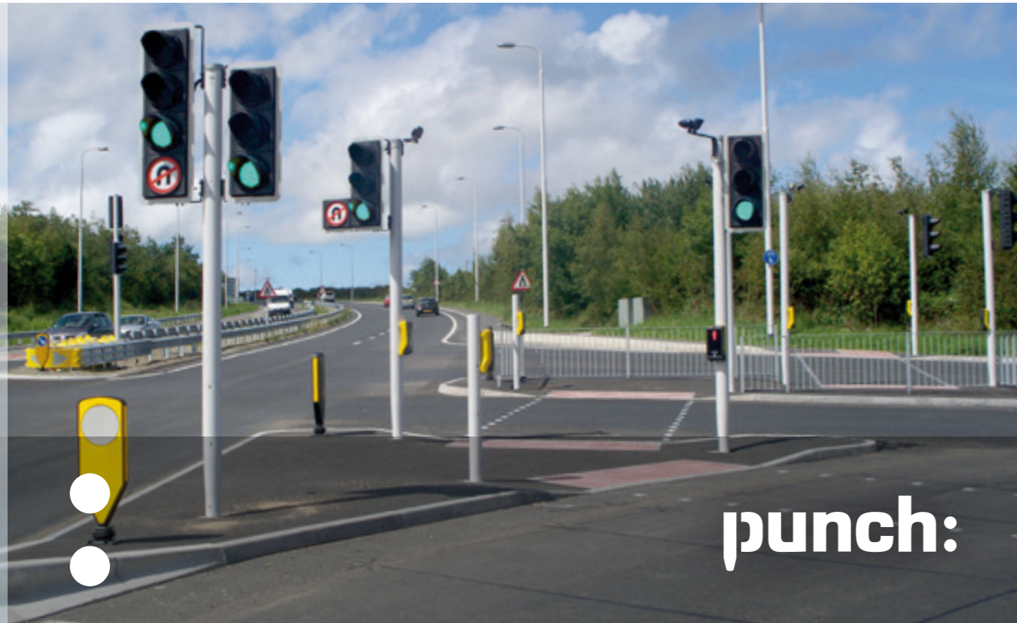
Traffic Signal Poles and push button poles
