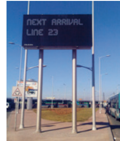
Support for Variable Message Sign
